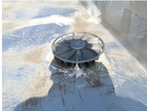
Treatment around the rainwater bucket
